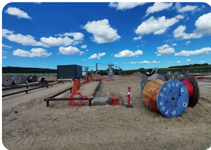
Battery park (BESS)
